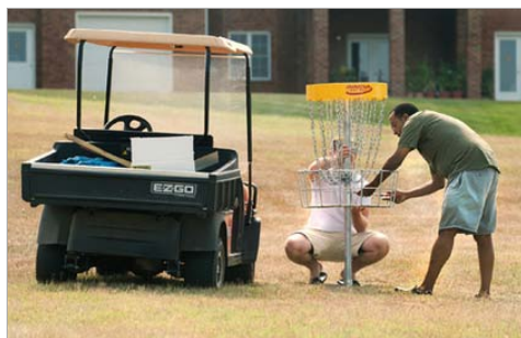
Zack Guida, a 2010 Bridgewater College graduate, and Teshome Molalenge, executive director of facilities support and auxiliary services at Bridgewater College, finish installing the last basket for a new flying disc golf course on Dinkel Avenue in Bridgewater July 30. (Photo by Michael Reilly)
